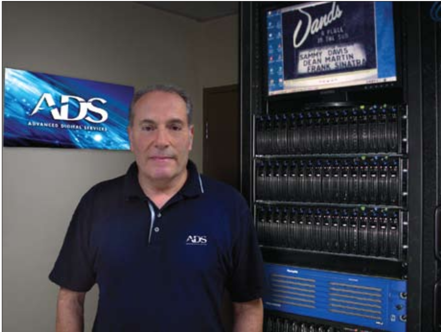
Russell Ruggieri, Advanced Digital Services' director of engineering, uses BlueStor PeSAN RAID arrays, which leverage the PCIe bus for host-storage connections.
